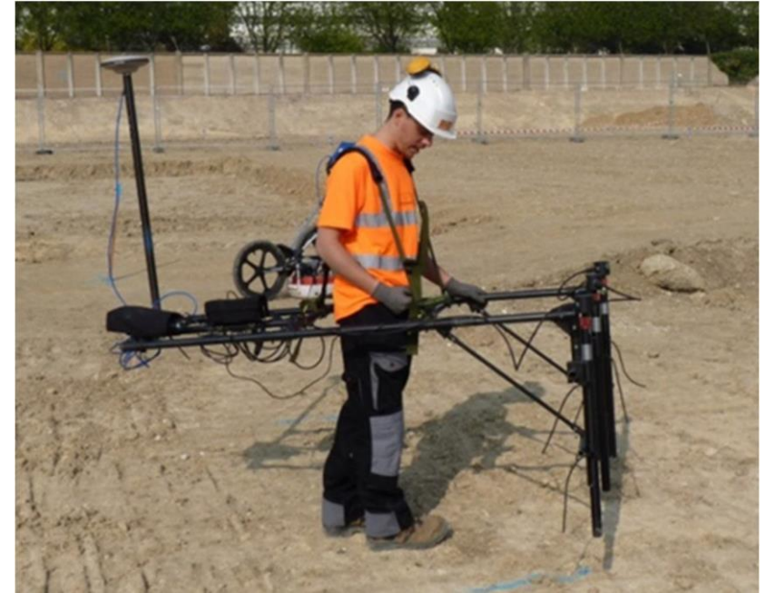
4 manually carried georeferenced probes mounting
